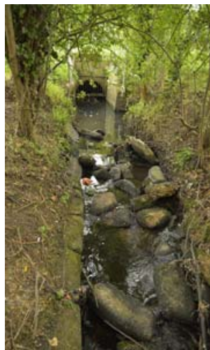
Shaded watercourse blocked with concrete
