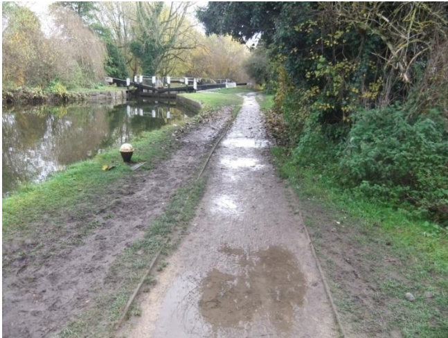
Figure 1 – Poor Towpath condition in Berkhamsted
